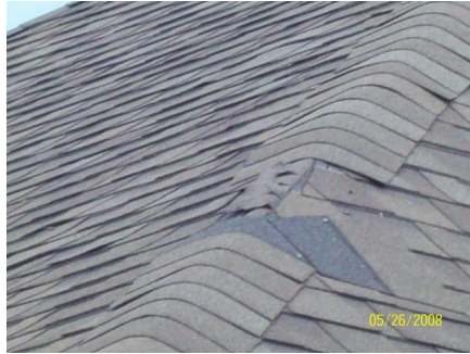
Damage shingles, northwest hip ridge
