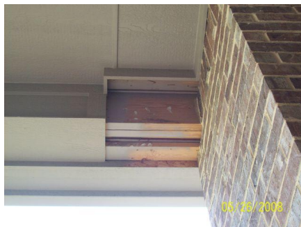
Missing cornice trim, front porch
