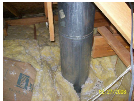
Insulation in contact with chimney flue
