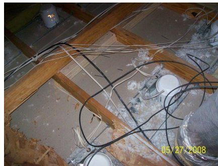
No insulation present above kitchen
