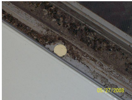
Sealant missing at window security contacts
