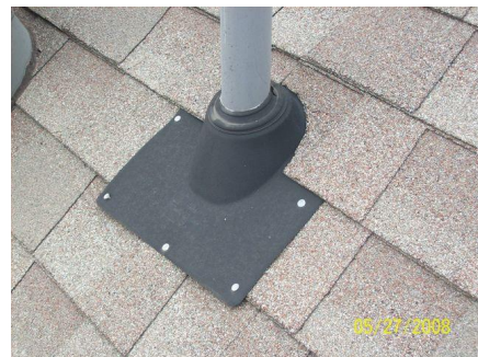
Exposed nail heads at vent boots
