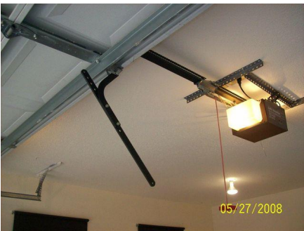
Operator not connected at garage door
