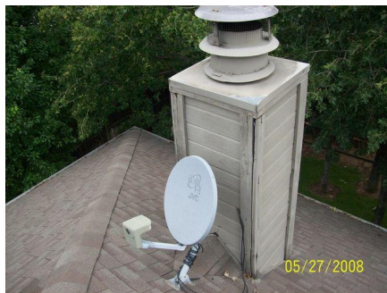
Wood trim water damaged at chimney
